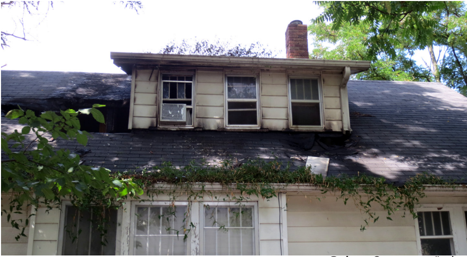
A hole burned through the roof of a house Aug. 29 on the 200 block of W. Normal St. The house suffered an estimated $30,000 worth of damage from the fire. Robert Overmann/Index
